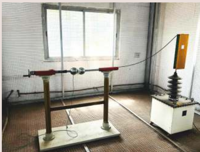
High Voltage Lab
